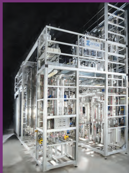
Two-stage hydroprocessing unit
