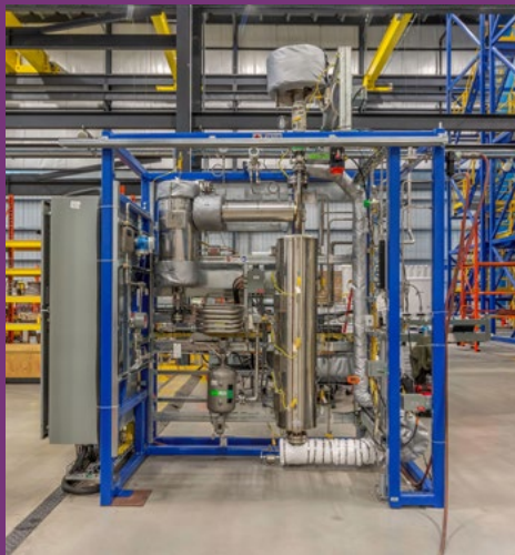
A fluidized bed calcination plant
