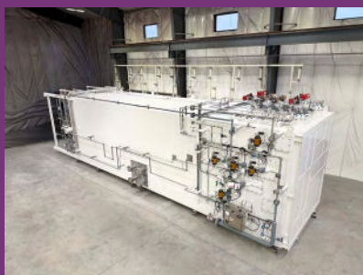
A hydrogen cryogenic adsorber system
