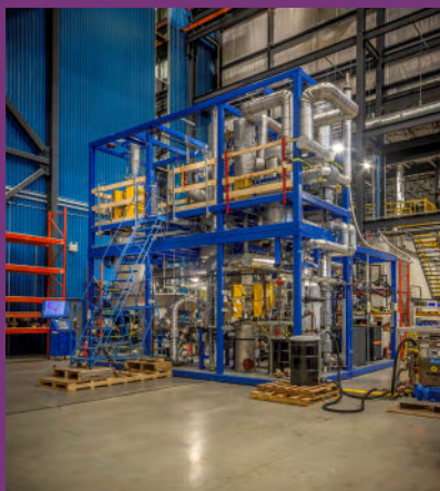
An insulation recycling pilot plant
