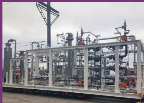
An industry-scale hydrogen deoxidation dryer system
