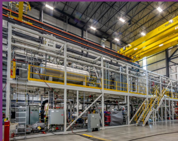
A large scale, high-pressure water electrolysis plant
