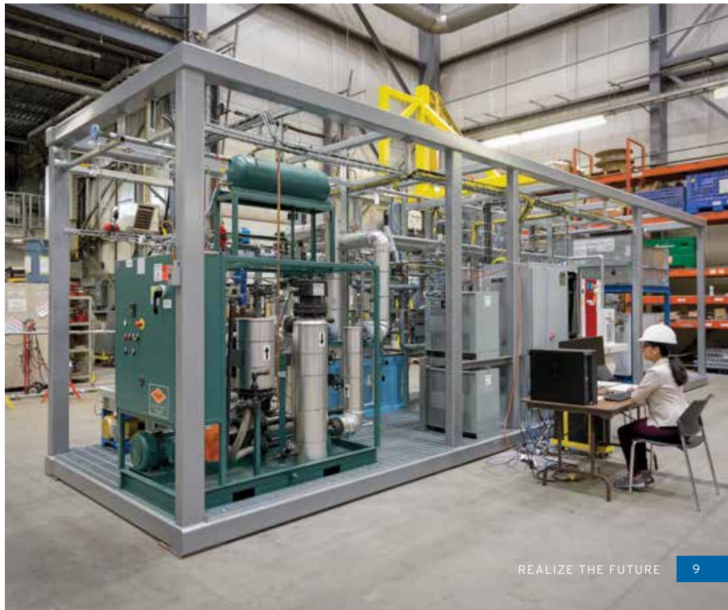
The 10x Scale Up Pilot Plant
