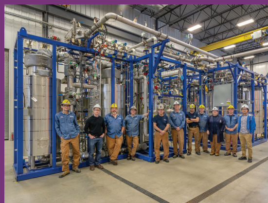
Five individual skid modules for a nuclear industry gas cleanup application
