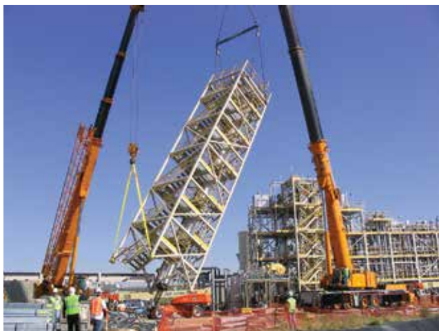
▲ Figure 1. Modular plants consist of steel frameworks (skids) on which process equipment, instrumentation, valves, piping components, and electrical wiring are mounted. The skids are transported to the construction site, where they are erected and connected to form the larger process system.
