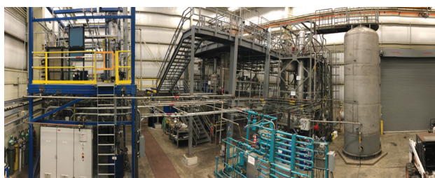
UK's Gasifier, Acid Gas Removal, and Syngas Compressor
