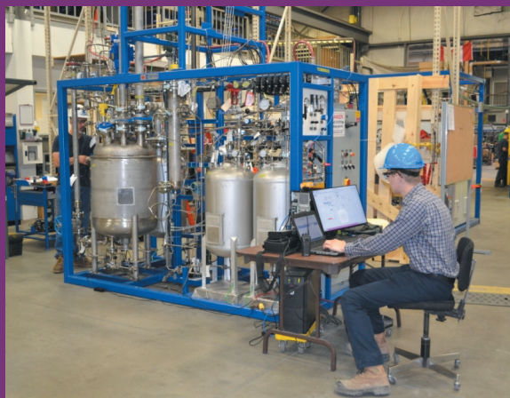
A pilot plant for specialty chemicals manufacture
