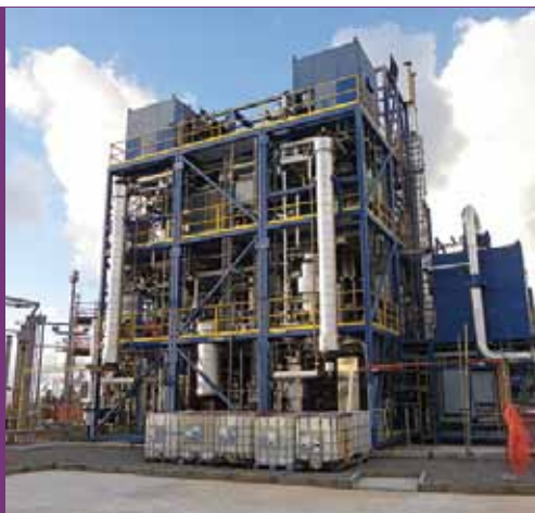
Gas-to-Liquids (GTL) demonstration plant for CompactGTL and Petrobras
