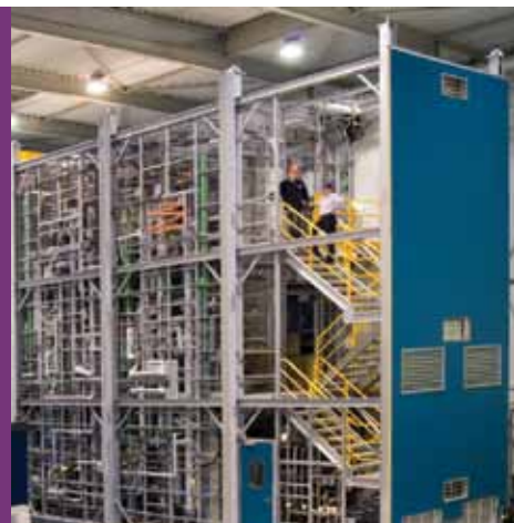
Enclosed outdoor chemical demonstration plant
