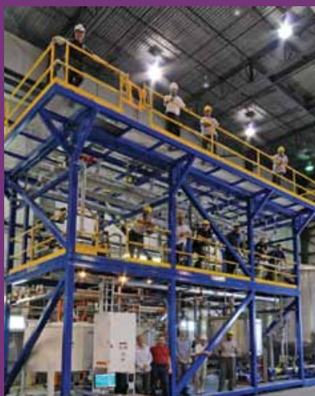
Azeo-Sep™ membrane plant for KMX Membranes
